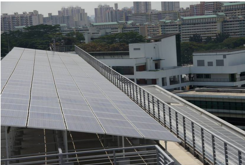
Solar panels on roof that reduces the carbon footprint of the Bosch Southeast Asia building
